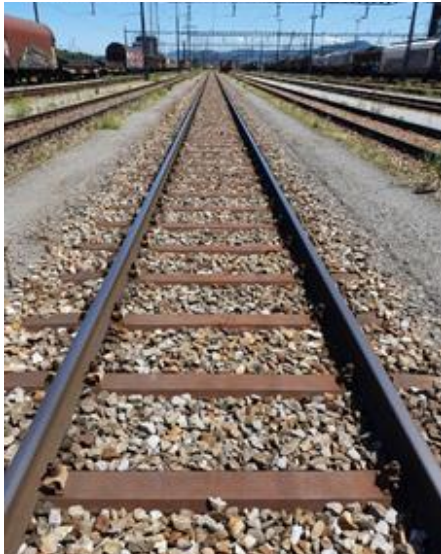
Figure 22: SBB Hot water case study - with hot water-maintained track (2 treatments)
